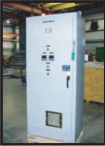
Heater Control Panel - Exterior
