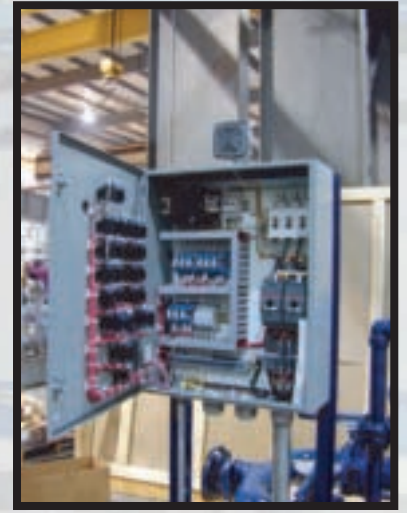
Integrated Systems Control Panel
