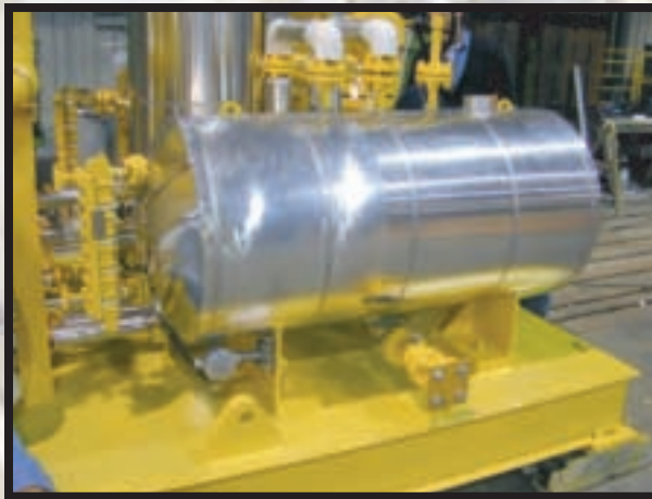
Detail: Hydrocarbon Drainage Tank
