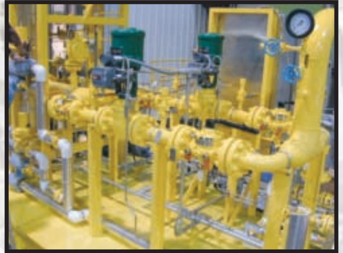
Detail Single Gas Path Pressure Reducing System
