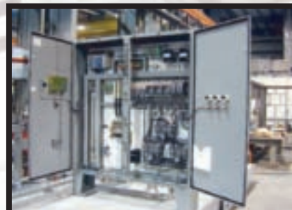
System Control Panel
