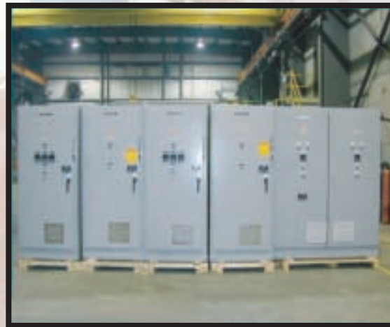
Various Heater Control Panels
