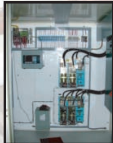
Detail: SCR Units, Controller
