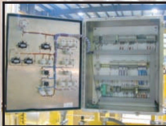
Integrated Systems Control Panel
