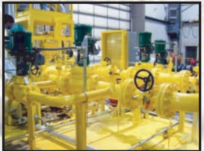
Detail: Dual Gas Path Pressure Reducing System
