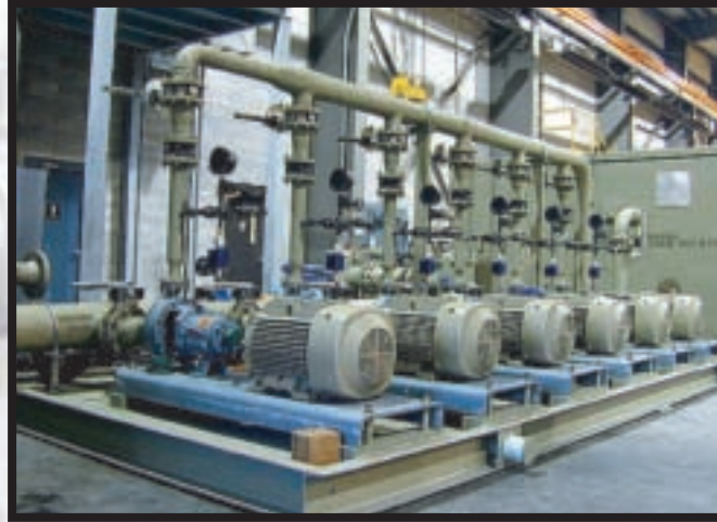
Liquid Process Pumping System
