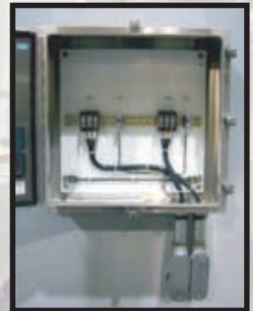
Motor Control Junction Box
