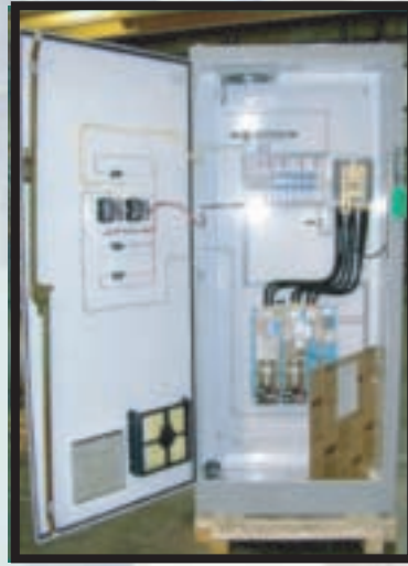
Heater Control Panel - Interior
