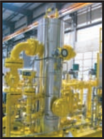
Detail: Knockout Drum
